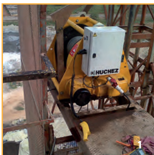
1. Lifting loads in a cement factory.
